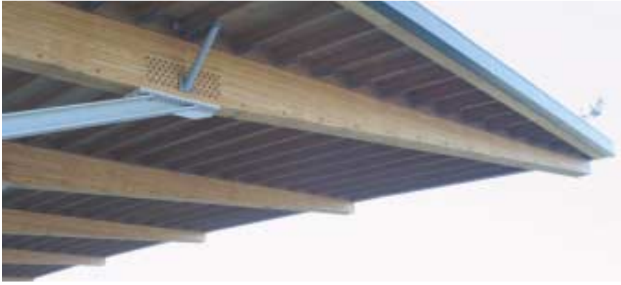
The glulam canopy was cambered, heightening the importance of accurate on-site fabrication and installation.
